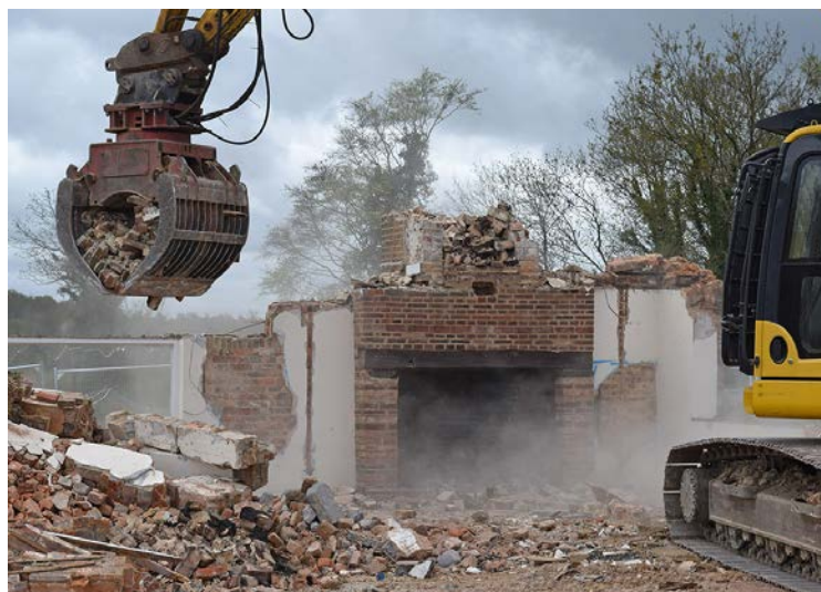
Supervised demolition of the farmhouse at Burgess Hill Farm after recording has been completed
